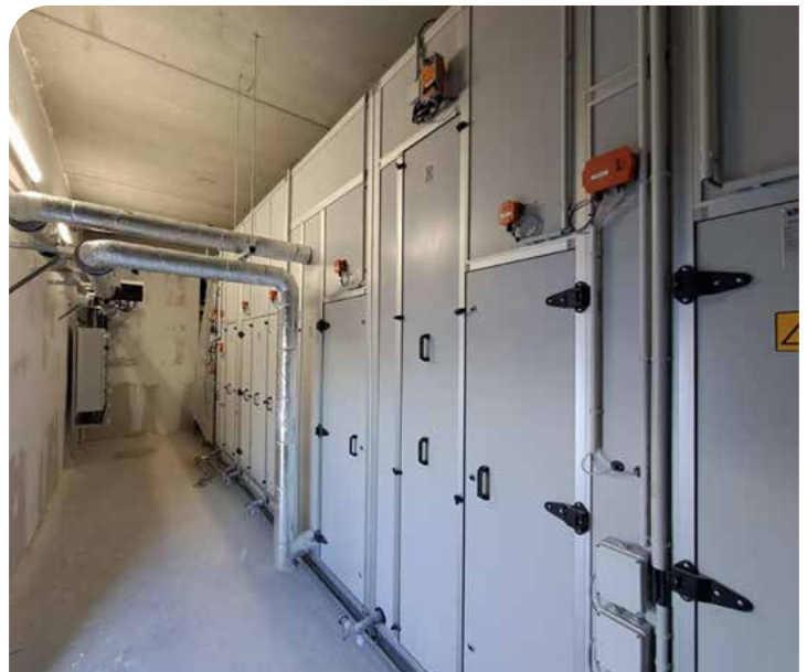
Air Handling Unit (AHU) for the Sarralbe swimming pool
